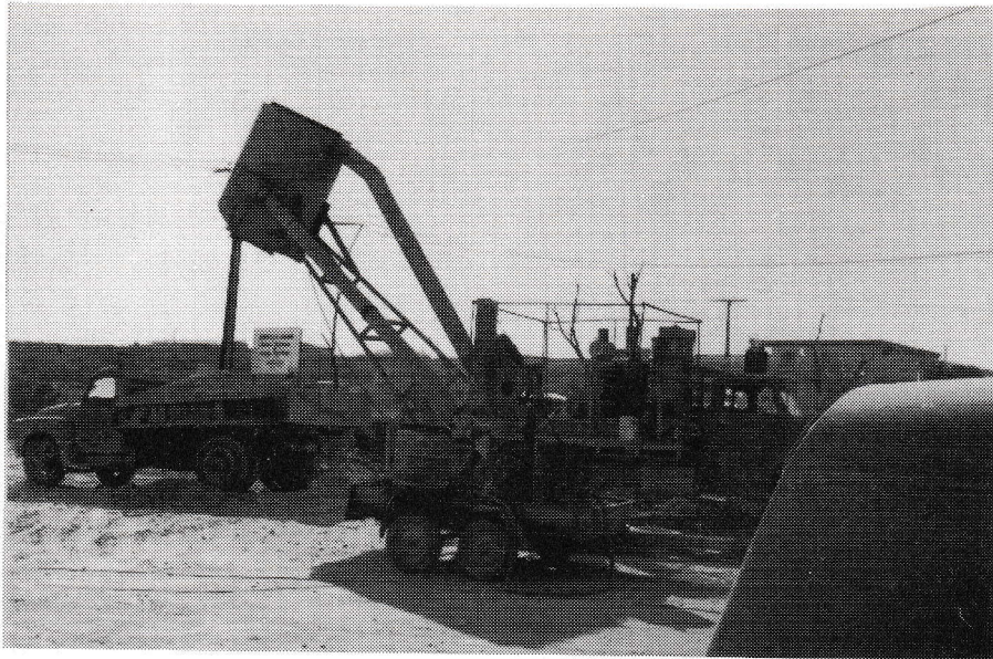
A BLOWER USED TO SHIFT THE ROCK AND DIRT FROM FROM THE DUGOUT.
