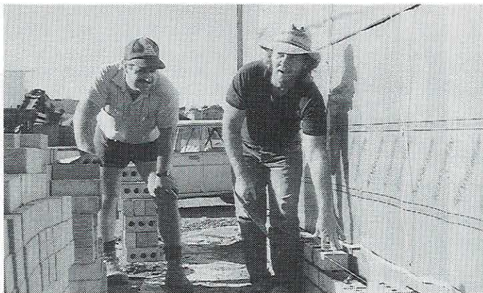
Works Manager Grant Drummond with brickie sub-contractor John Spasojevic laying the first course on the new depot offices
